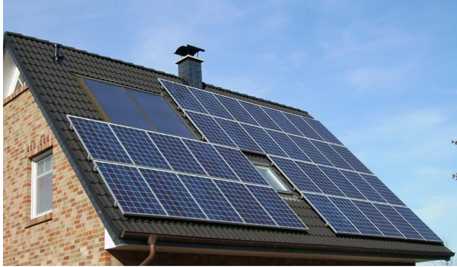
Fig. 3.5 Solar panels on roof
