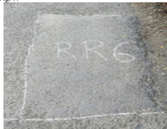
Fig. 9: Sample Patching on RR-6
