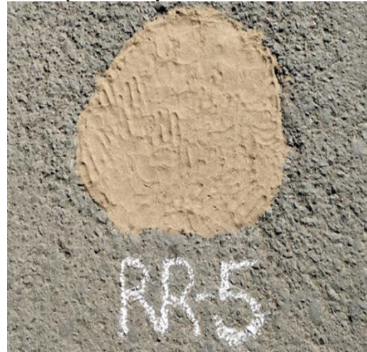
Fig. 8: Volume Determination by Replacing Sand with Bowl of Pothole
