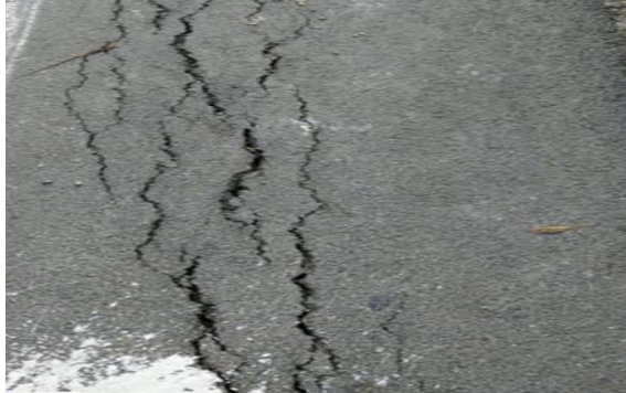
Fig. 10: Sample of Longitudinal cracking
