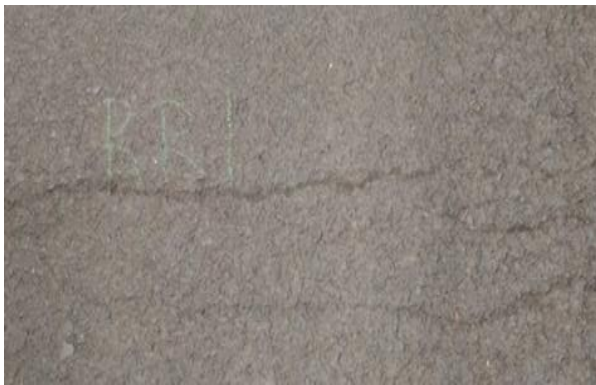
Fig. 11: Sample Transverse cracking
