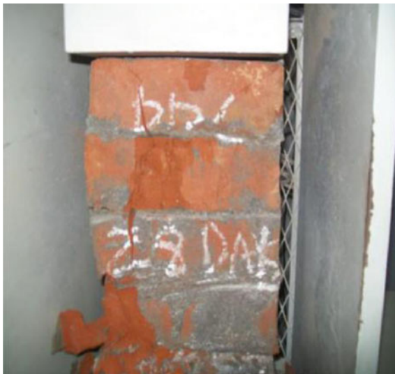
Fig. 9 Unconfined masonry failure
