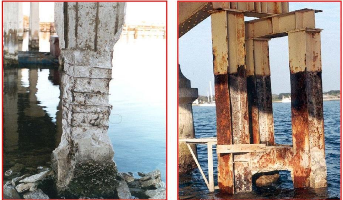
a) Degraded concrete pile
