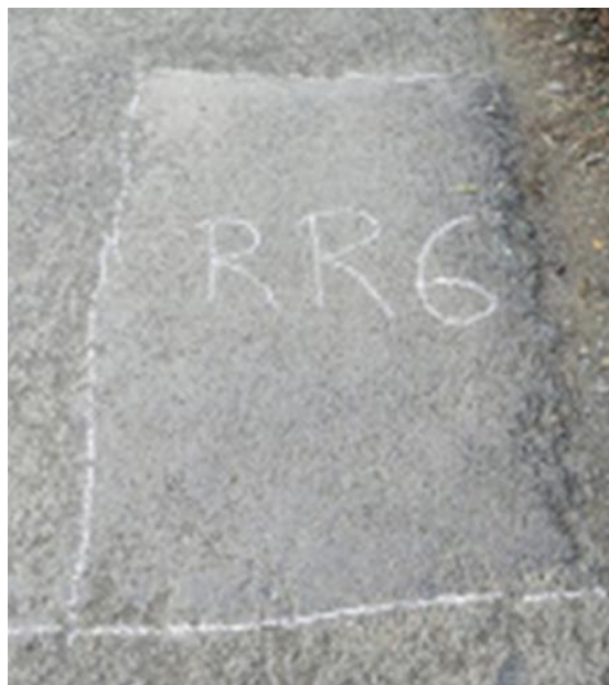
Fig.4.6: Patching at RR-6
