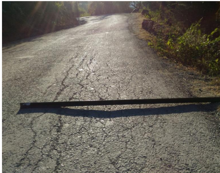
Fig.1.2: Rutting on the road surface
