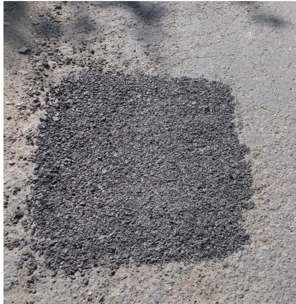
Fig.1.4: Patching at RR-1
