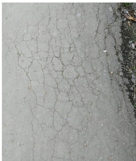
Fig.4.9: Alligator cracking at RR-1
