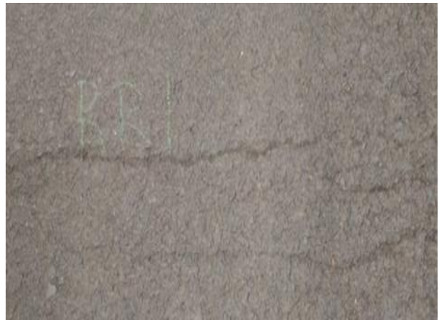
Fig.4.8: Transverse cracking at RR-2
