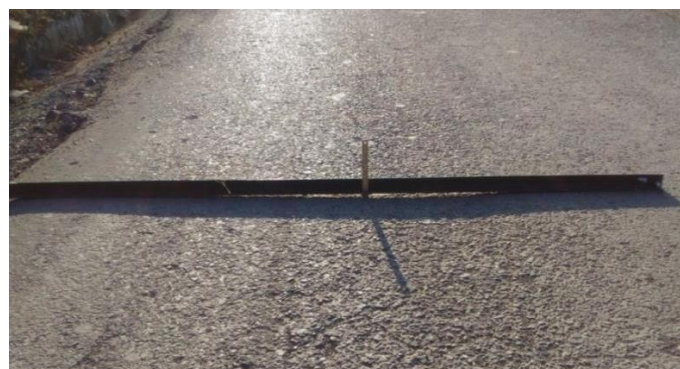
Fig.4.4: Rut depth on pavement
