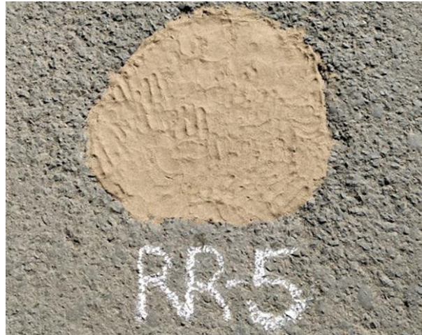
Fig.4.5: Determining volume of pothole at RR-5
