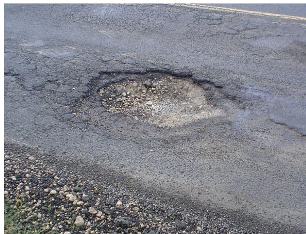
Fig.1.3: Depression due to pothole
