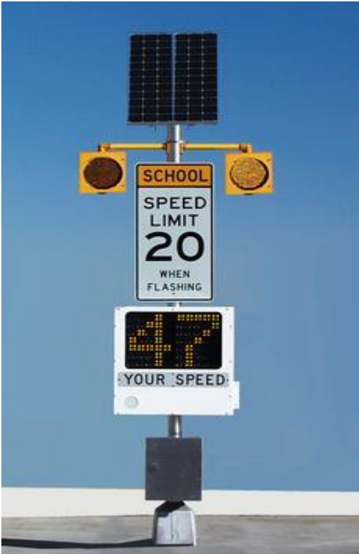
Figure 4.2: Lights and sensors running by solar panel [15]
