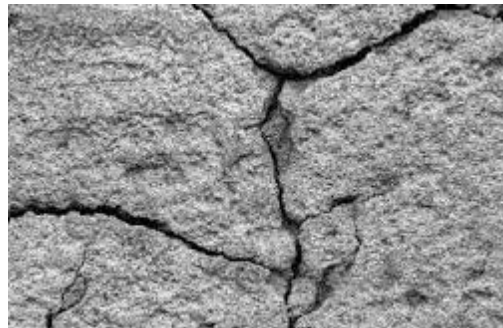
Figure 4: Concrete Crack Failure
