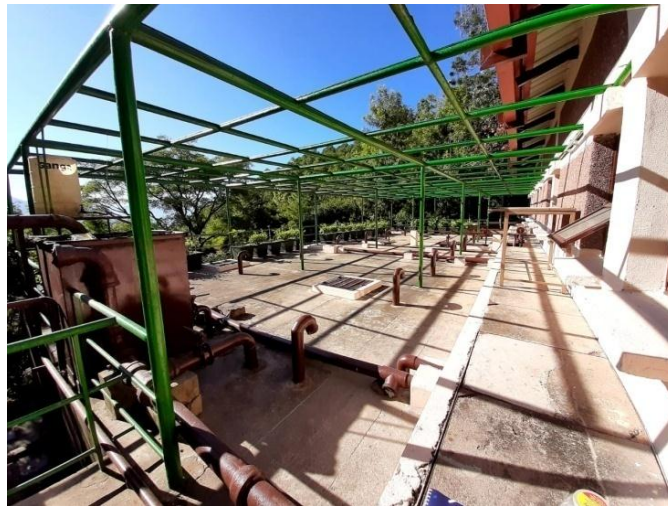
Figure 1.2 Typical view of STP
