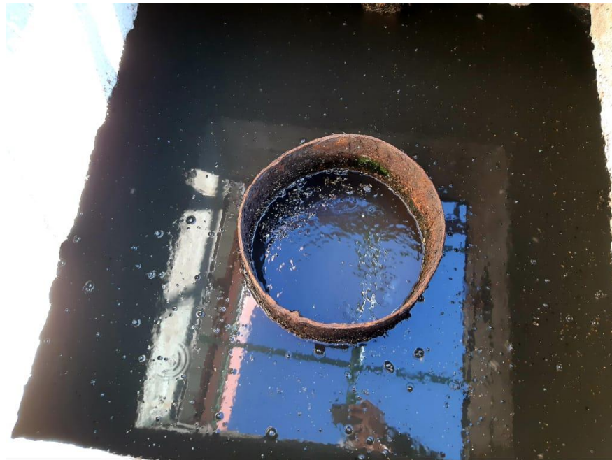
Figure1.5 Sludge tank of STP
