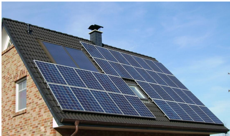
Fig. 3.5 solar panels on roof
