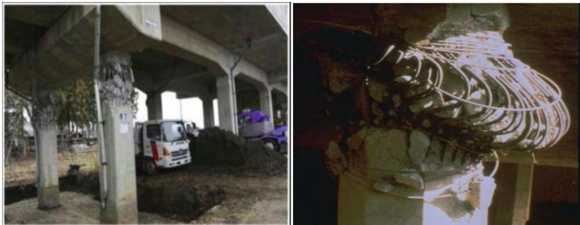
Fig.1.1 Failure of column
