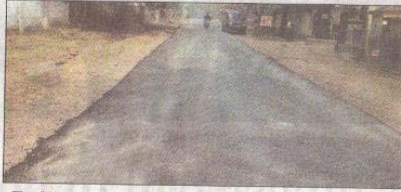
The 400-foot stretch of a road using plastic waste in the Circuit House area of Jamshedpur.
