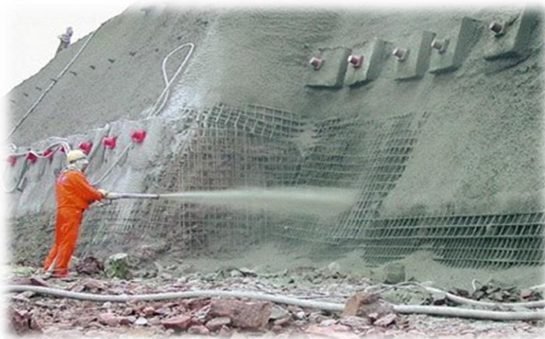
Fig 1.6: Shotcreting is done with the help of a pipe with a nozzle
