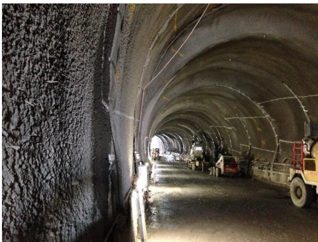
(Fig.1.4) Innovative Use of Fiber Reinforced concrete on The North Strathfield Rail Underpass
