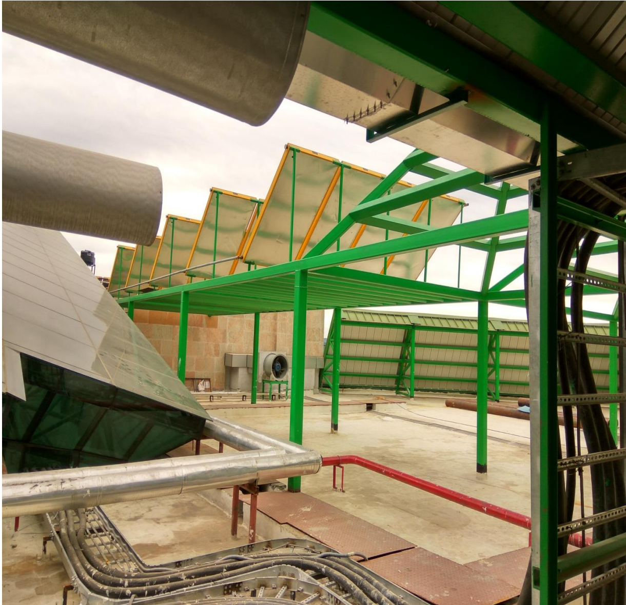
Fig.4.2 Solar Window and Roof window used in SJVNL for Energy Efficiency
