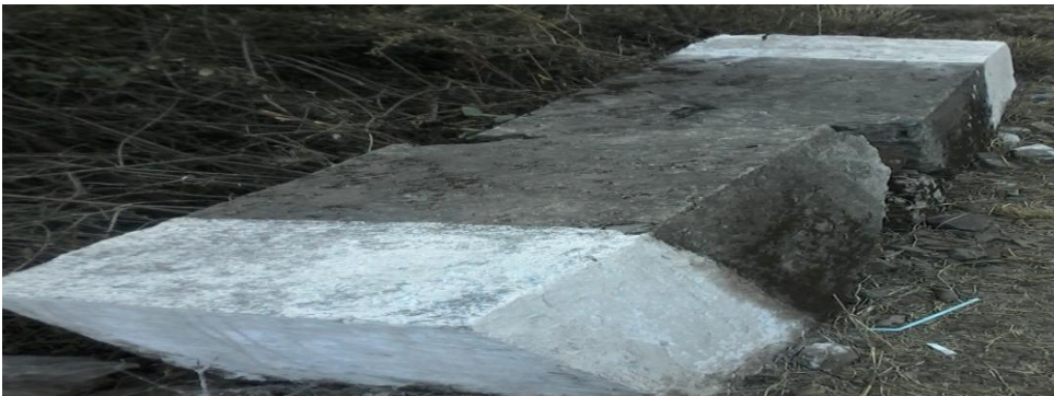
Fig 5.9 Condition of parapet is not good .
