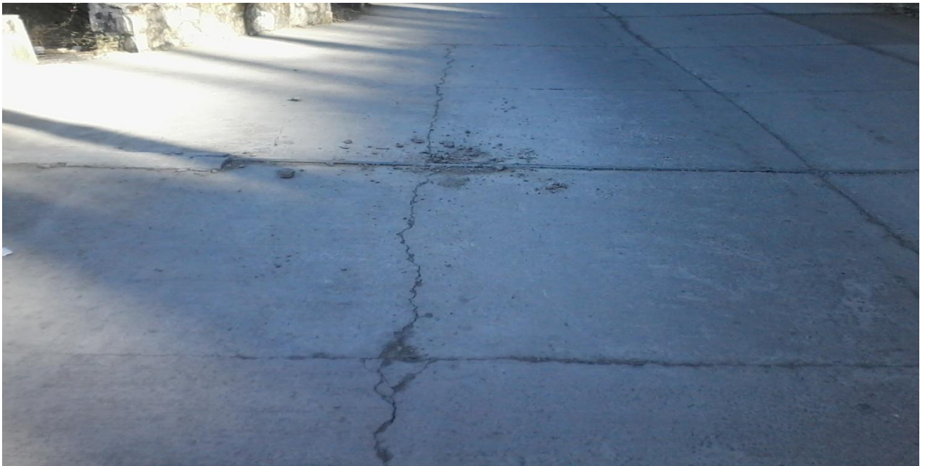
Fig 5.3 (e) Condition of the concrete pavement is not good
