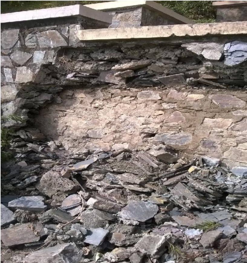
Fig 3.2 Delaminated wall near the play ground
