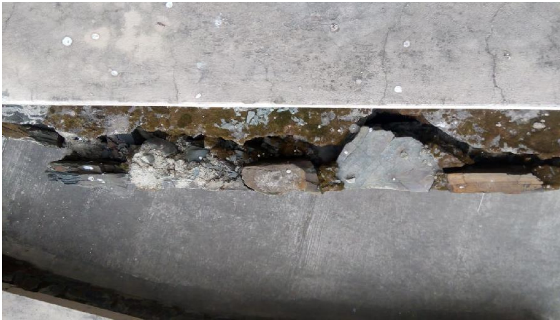
Fig 2.1 and 2.2 Top view of the cracks in shear wall
