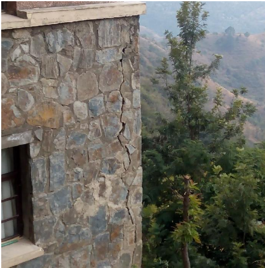
Fig 2.3 and 2.4 Cracks in the column of C4 block.
