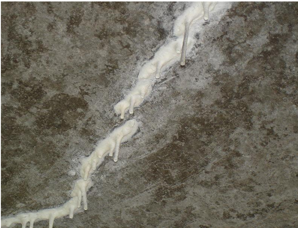
Fig 1 white scales with water percolating from it on the roof of ECE department
