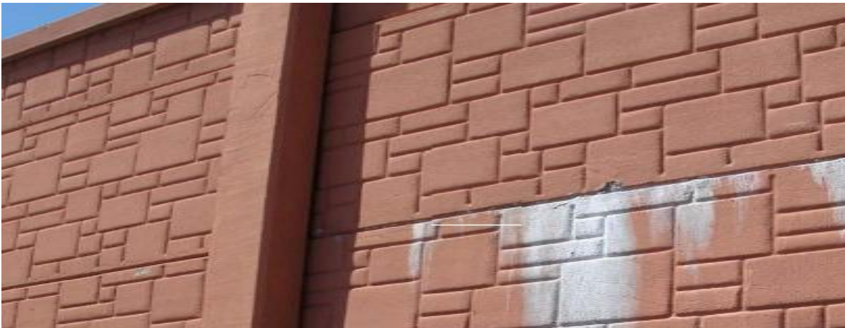
Fig 1.3 Lime boom efflorescence
