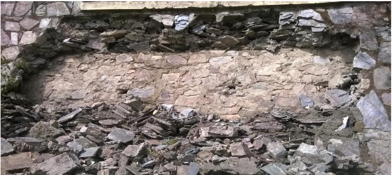
Fig 3.1 front view of the delaminated wall
