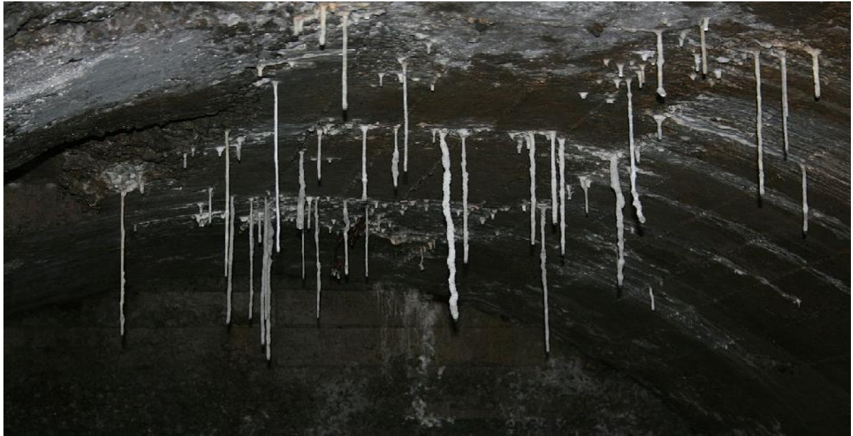
Fig 14 Lime weep efflorescence
