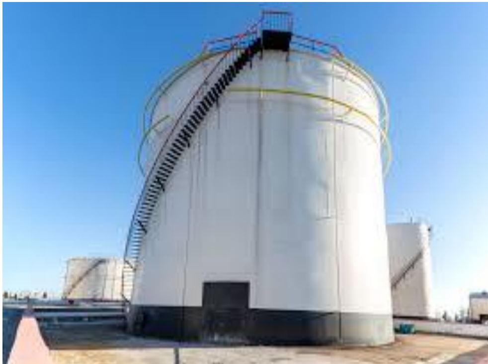
Figure 1.2(a) Aboveground storage tank [9]
