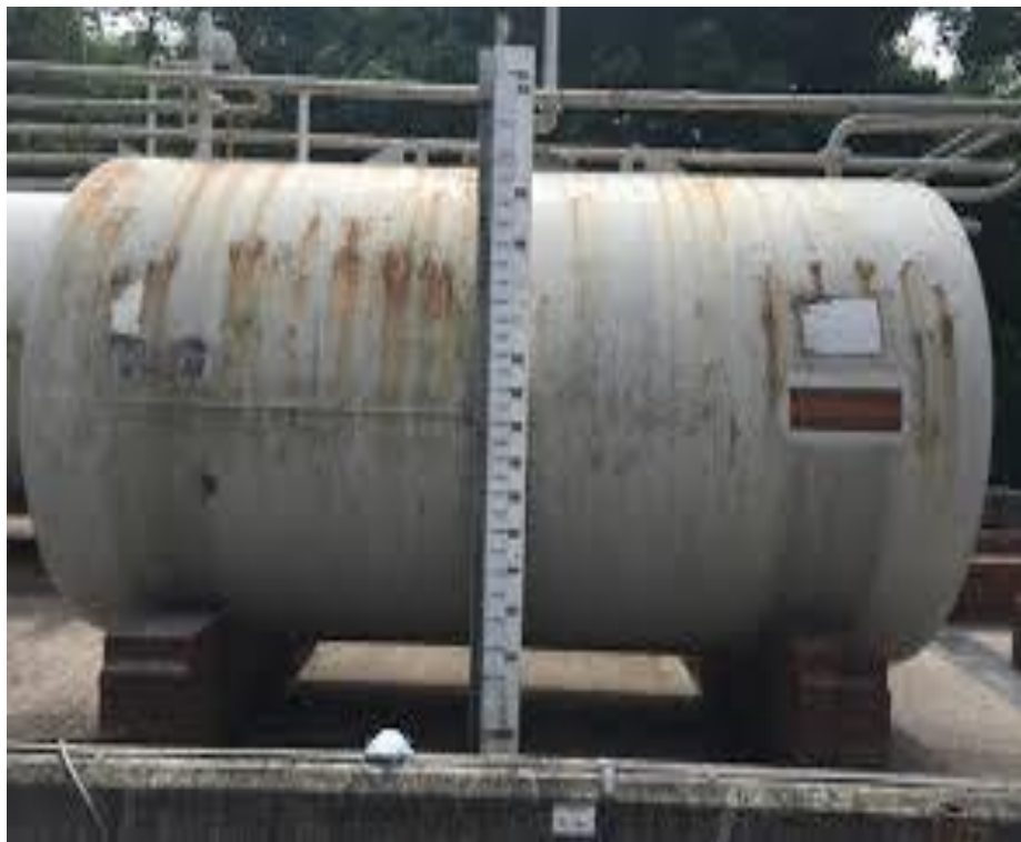
Figure 1.5 Corrosion taking place in a tank [12]
