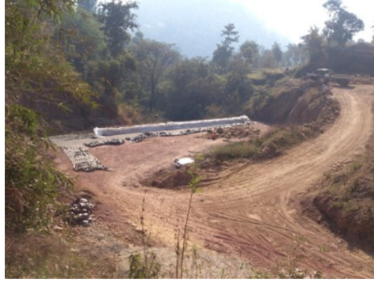
Geotextiles placed perpendicular to the surface and geogrids placed parallel to the surface
