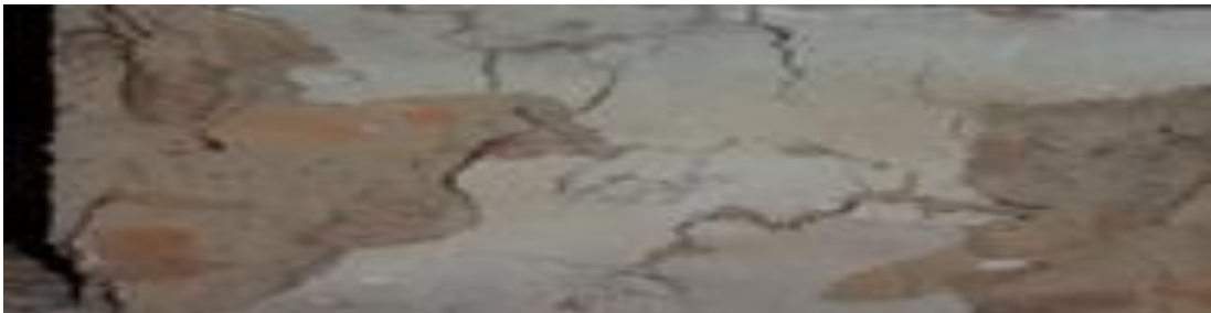
Fig 8: Pictures showing change in colour of concrete
