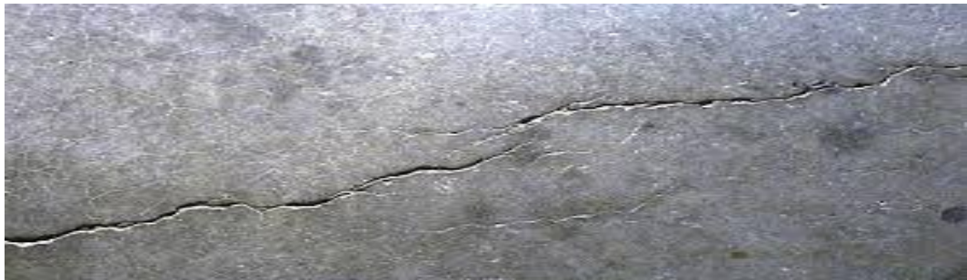
Fig 9: Pictures showing surface cracks
