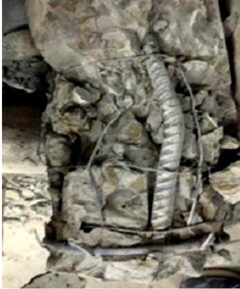
Figure 4.10 Failure of 4RWS
