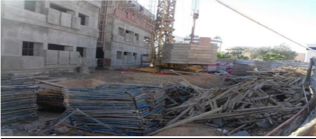
Fig.3.2 - Poorly organized construction site
