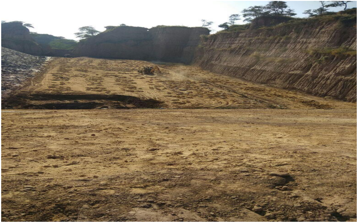
Figure 13 Dumping area of Shivalik Solid Waste Management Plant
