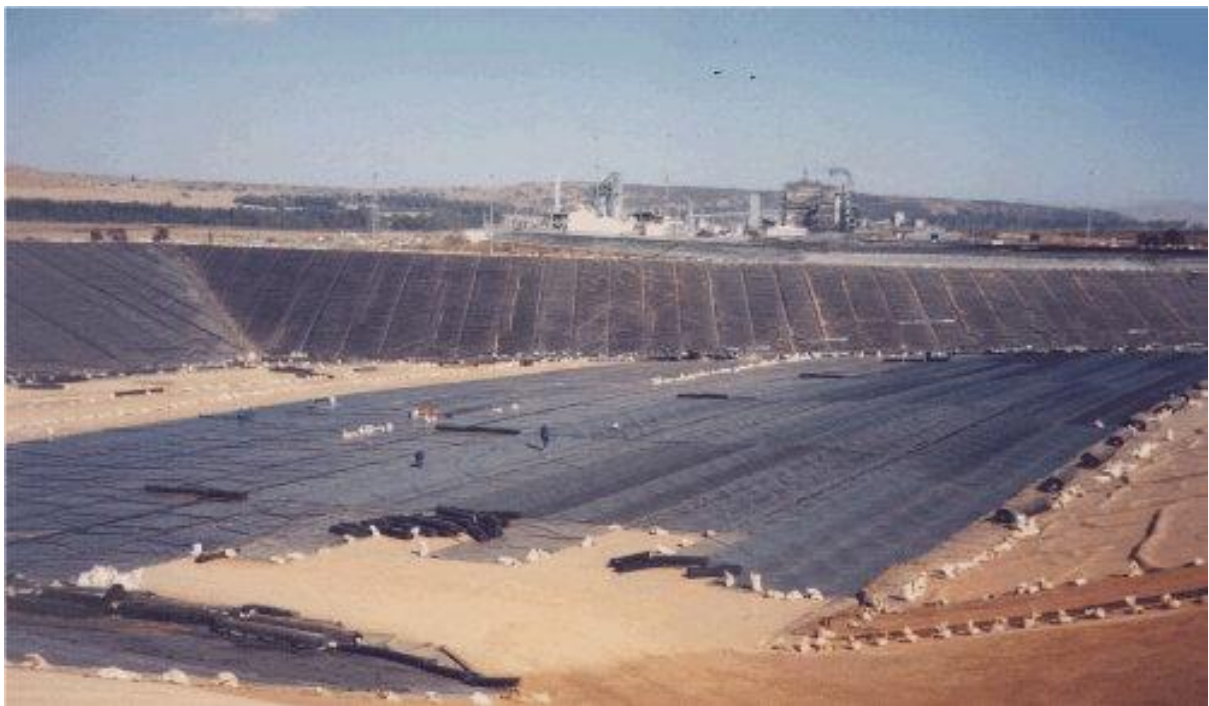
Figure 8 Nimbua Green Field Dump Site
