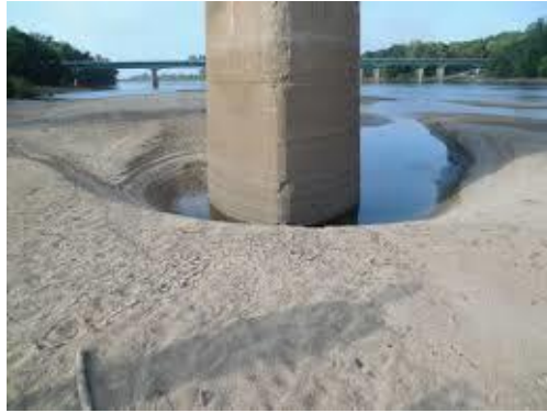
Fig.12 Scour Around Pier
