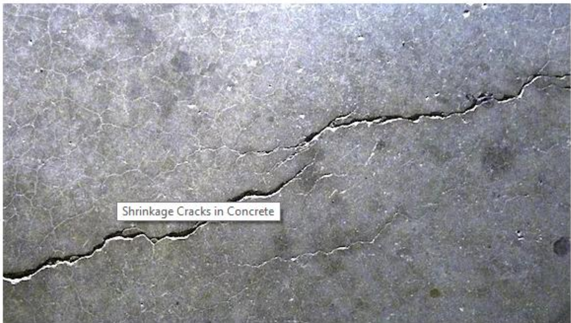
Figure 3.7 Shrinkage cracks in concrete
