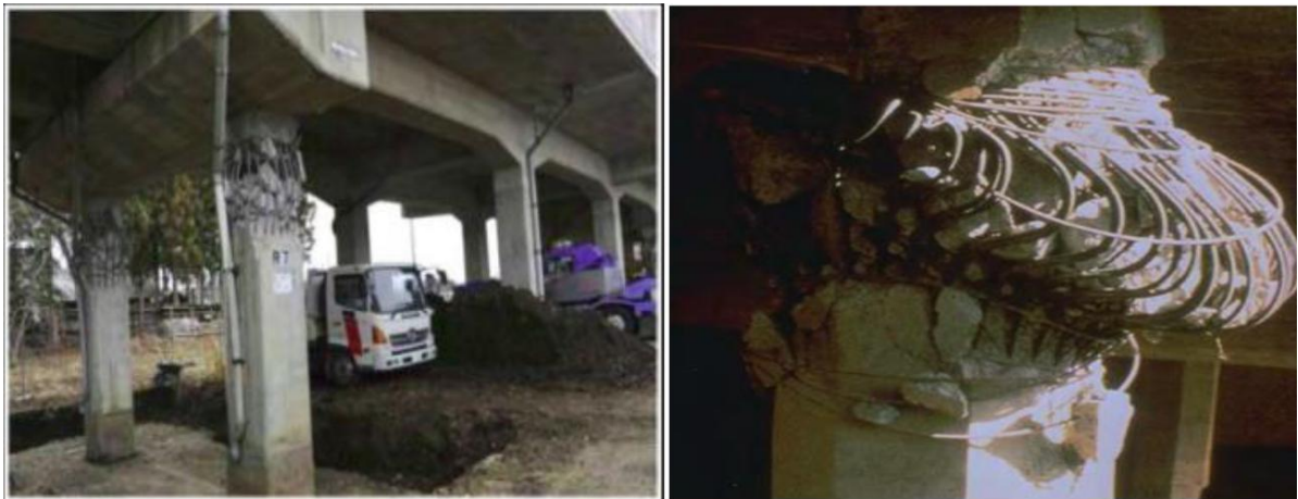
Figure 1.1 Failure of concrete due to lack of confinement
