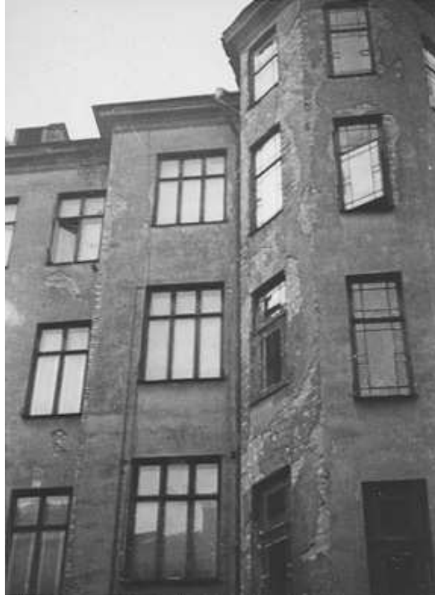
Figure1. Dilapidated house in the back garden on Karlaplan 4.
