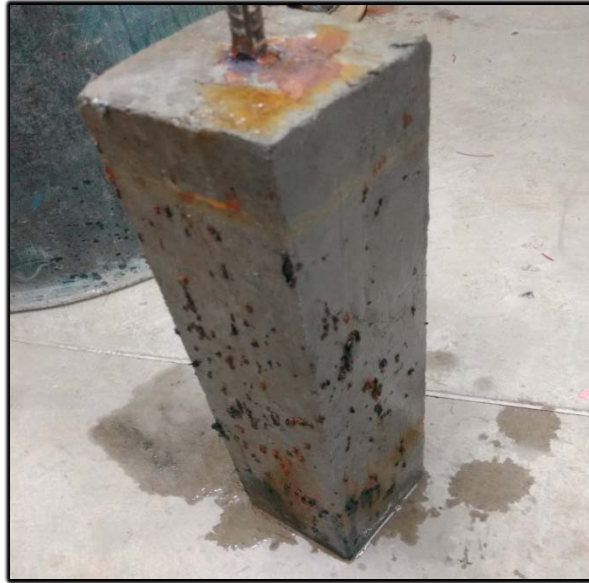
Figure 4.4: Staining due to steel fiber corrosion.
