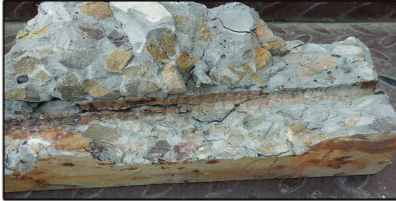
Figure 4.9: Corrosion depth of the concrete samples
