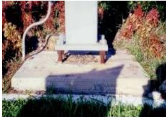
Fig. 1.2: Utility pole at a park [1].
