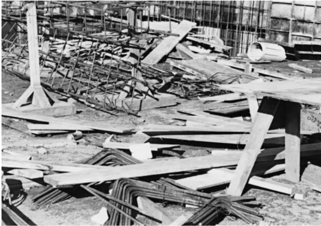
FIGURE 2.2 An unsafe/congested work area
