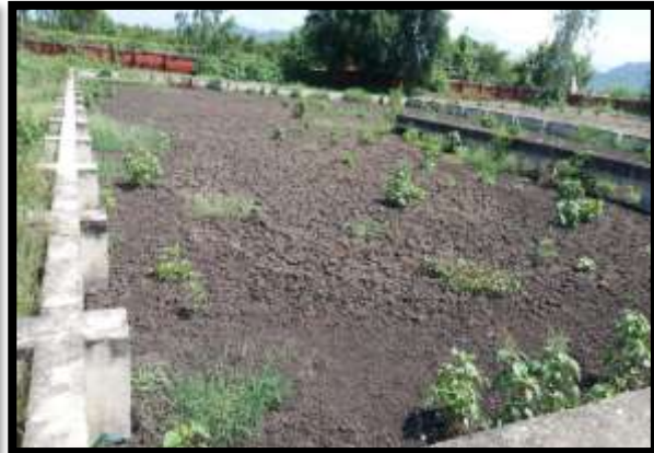
Fig. 3.4 Sludge Drying Pans
