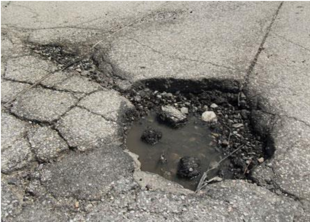
Fig. 1-Pavement Deterioration (Pot Hole)
