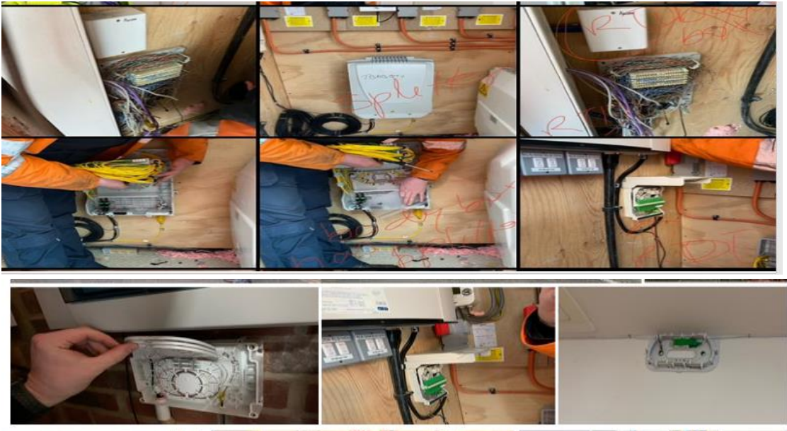
Fig 2.3.2.2 Real Equipment at the site
