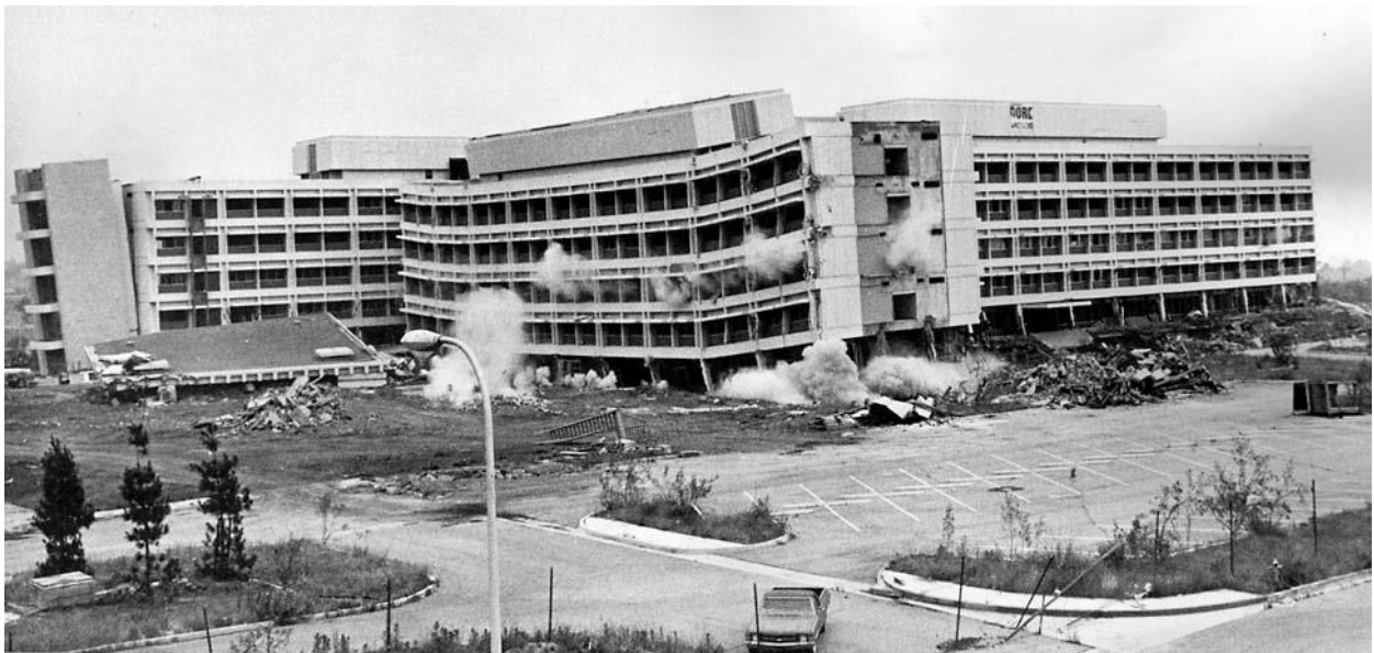
Figure 4 1971 Earthquake Damage of Olive View Hospital
