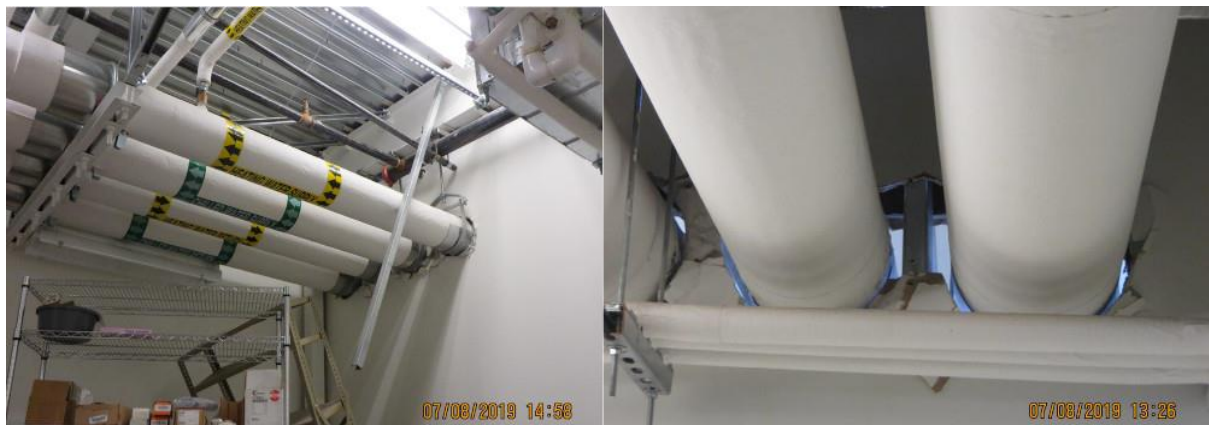
Figure 7 Damage to water supply pipes in Ridgecrest healthcare facility.
